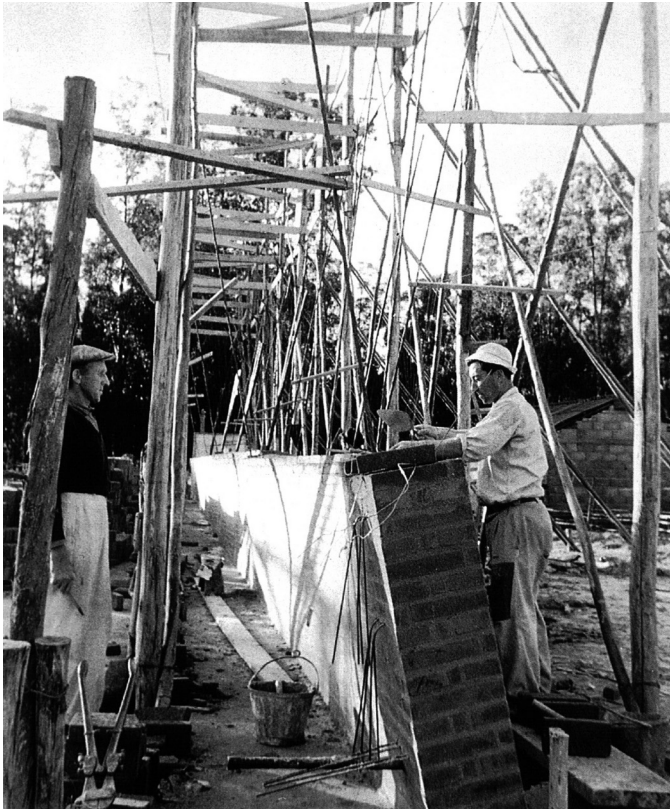
Figure 1: Construction of ruled surface walls at Church of Christ the Worker in Atlántida, Uruguay. Image from Dieste Archive published in Remo Pedreschi's, The Engineer's Contribution to Contemporary Architecture .
