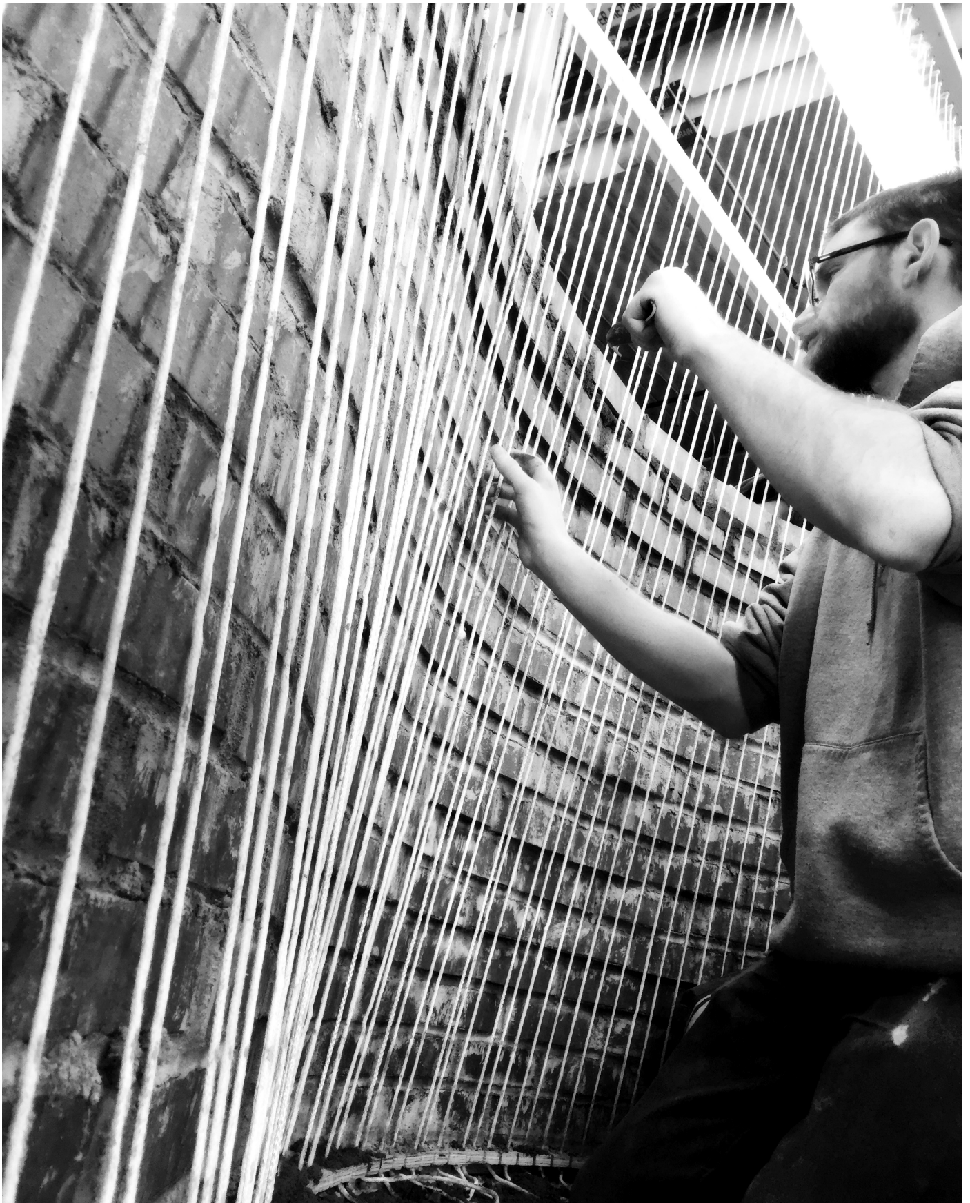
Figure 5: Ruled surface brick wall construction. Curved Walls: Eladio Dieste and Ruled Surfaces Workshop, South Dakota State University.
